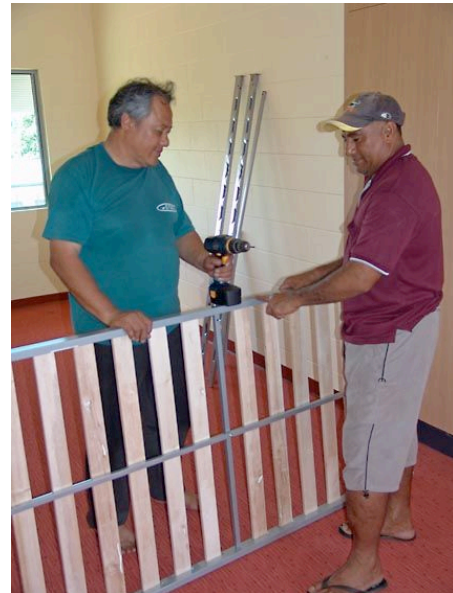
Malofau Chan Foon & Laupisi Asi fitting out the new residence on the school property
